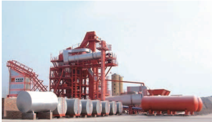
Type 4 – “Double Drum” series (adding RAP into a separate drum dryer)
